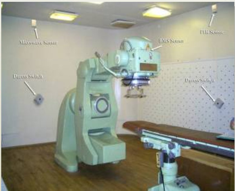
Oncology clinic security enhancements include installation of sensors to detect entry into room that holds source and sensor on the teletherapy unit itself.
