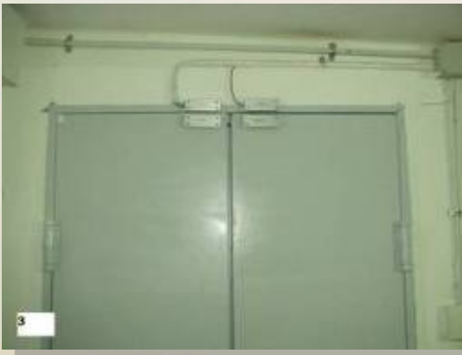
Interior Intrusion Detection
