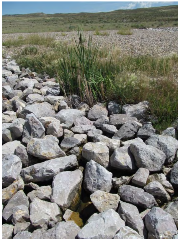
MAY 8/2013. PL-8. Cattails growing adjacent to the base of the east side slope of the disposal cell; standing water within apron in foreground.
