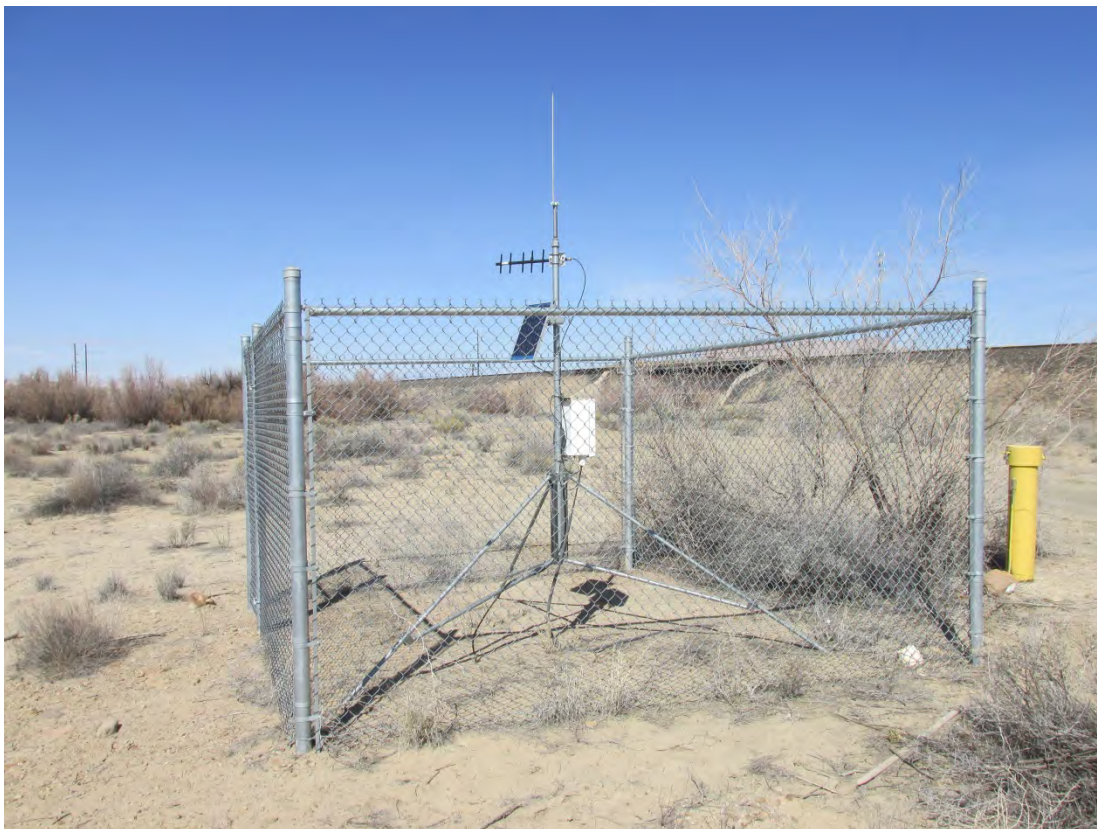
GRN 3/2013. PL-3. Enclosed telemetry station at monitoring well 0817.
