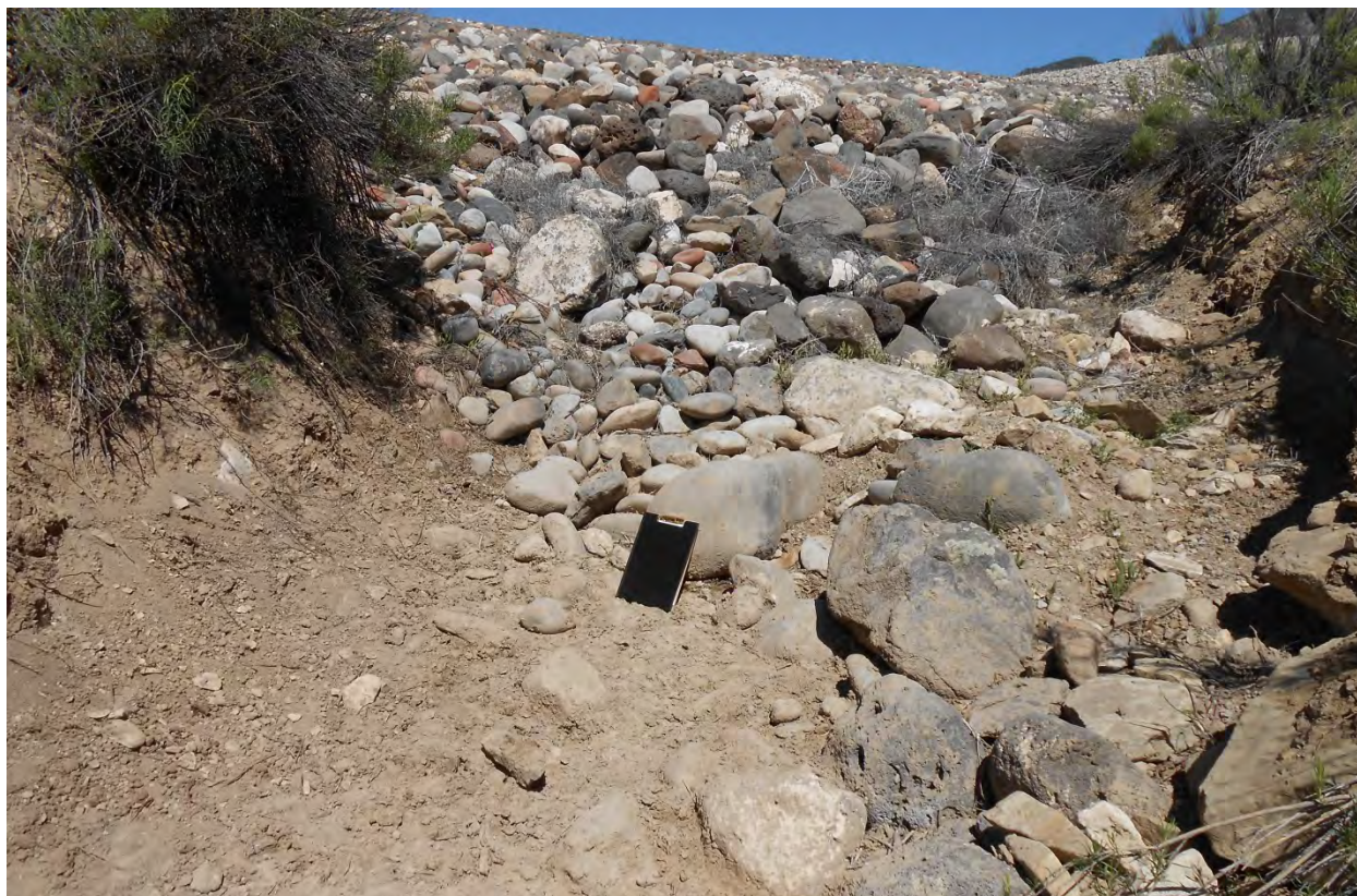
RFL 6/2013. PL-8. Evidence of cattle at toe ditch runoff point.
