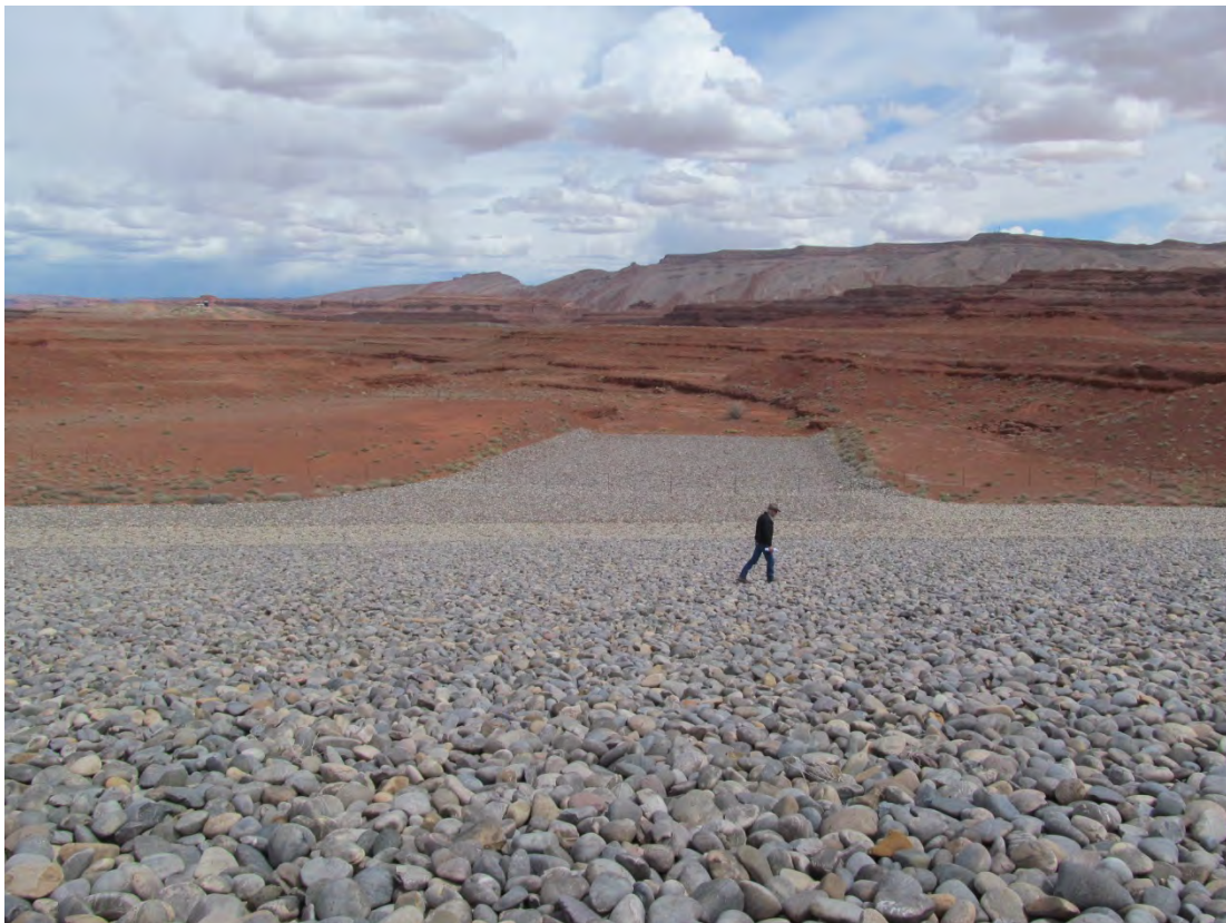
HAT 4/2013. PL-8. Northeast toe drain.
