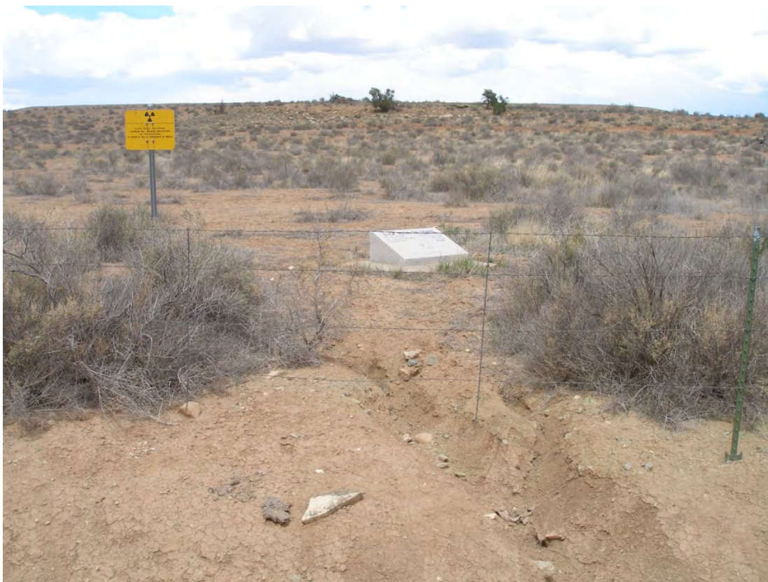
SRK 5/2013. PL-1. Site marker near entrance gate, erosion
