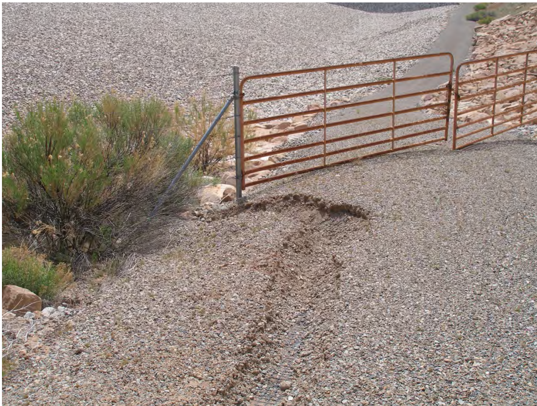
NAD 5/2013. PL-2. Erosion on access road near upper gate.
