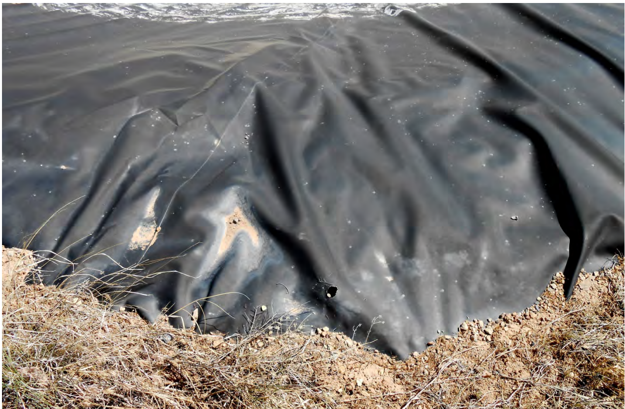
RFL 6/2013. PL-7. Small hole in evaporation pond liner.
