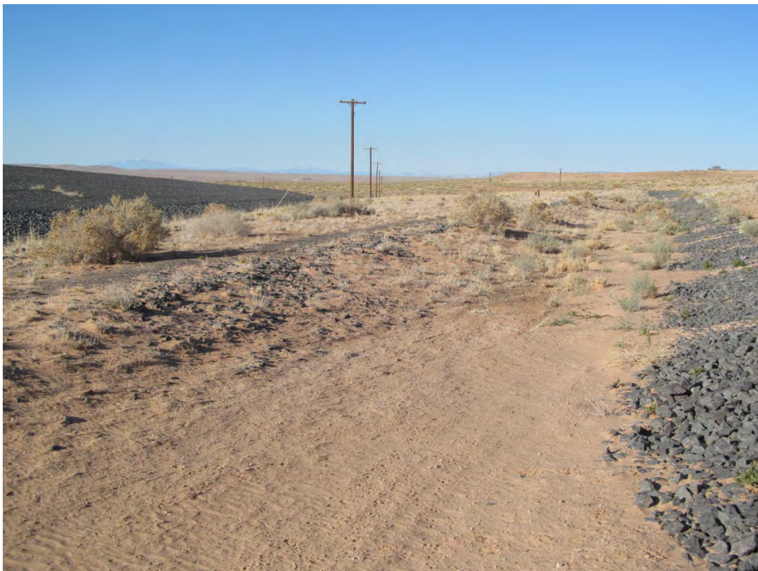
TUB 4/2013. PL-11. West of footbridge showing sediment in channel.
