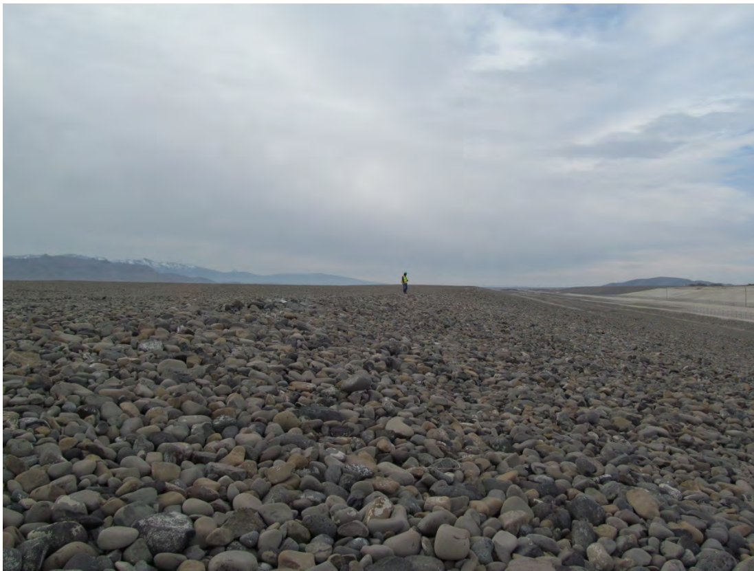
SLD 3/2013. PL-6. UDEQ personnel illustrating unevenness of the ridge construction along the top of the west slope.
