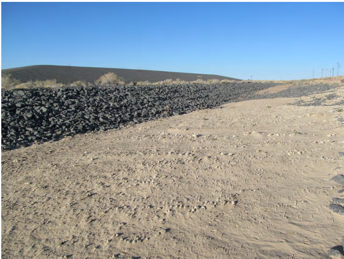
TUB 4/2013. PL-13. West along base of channel (revegetation and washout).
