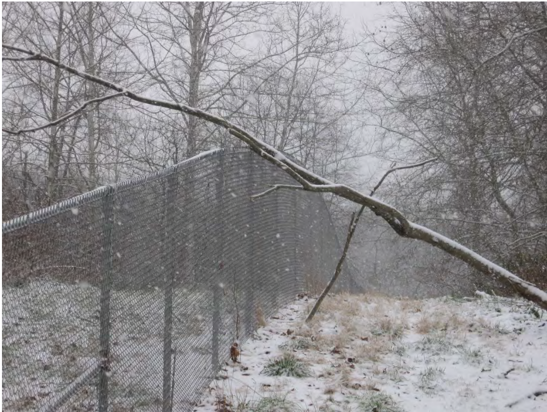
BUR 12/2013. PL-2. Tree down on south fence.
