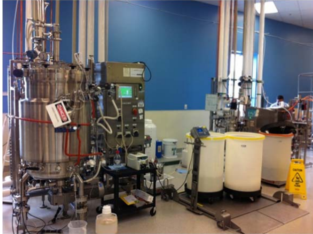
Figure A.8: Fermentor F3 in Operations after February 2011 commissioning
