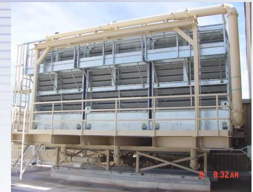
Cooling Water Tower
