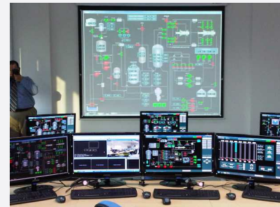
Reactor Analysis, Design and Instrumentation Controls Lab
