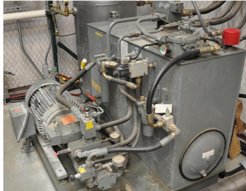
Existing 25 hp Hydraulic Power Unit at Sandia
