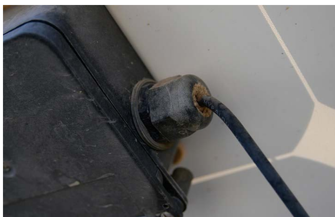
Fig. 3. Example of an aged connector at the Distributed Energy Technology Laboratory at Sandia National Laboratories that can be later used to correlated acceleration factors with actual degradation rates in the field.
