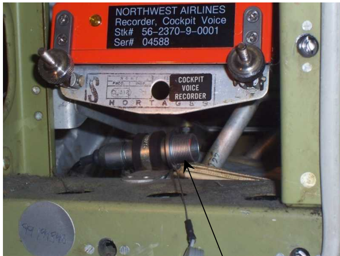
TPS connector routed to access panel
