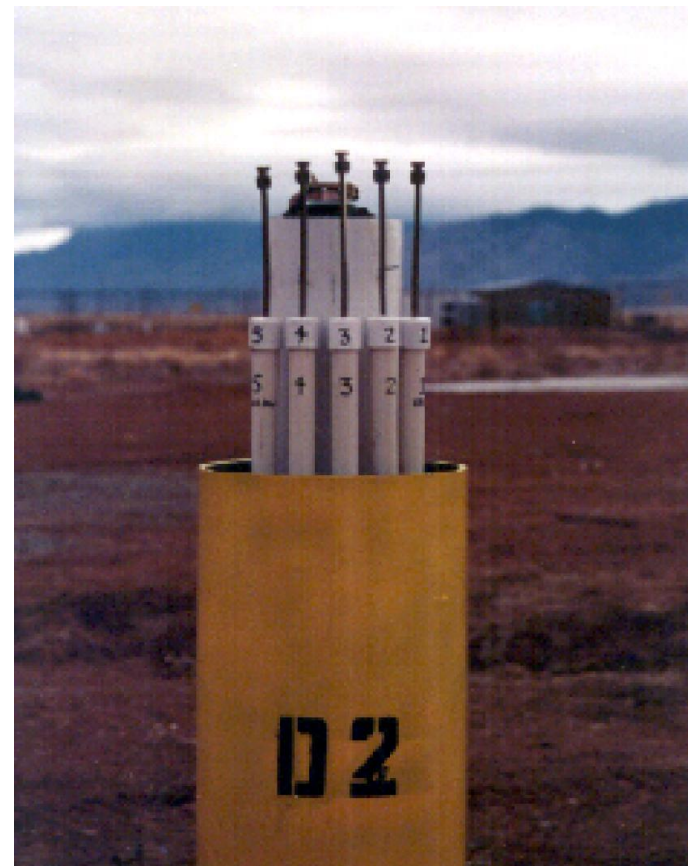
Vapor Extraction System Well
