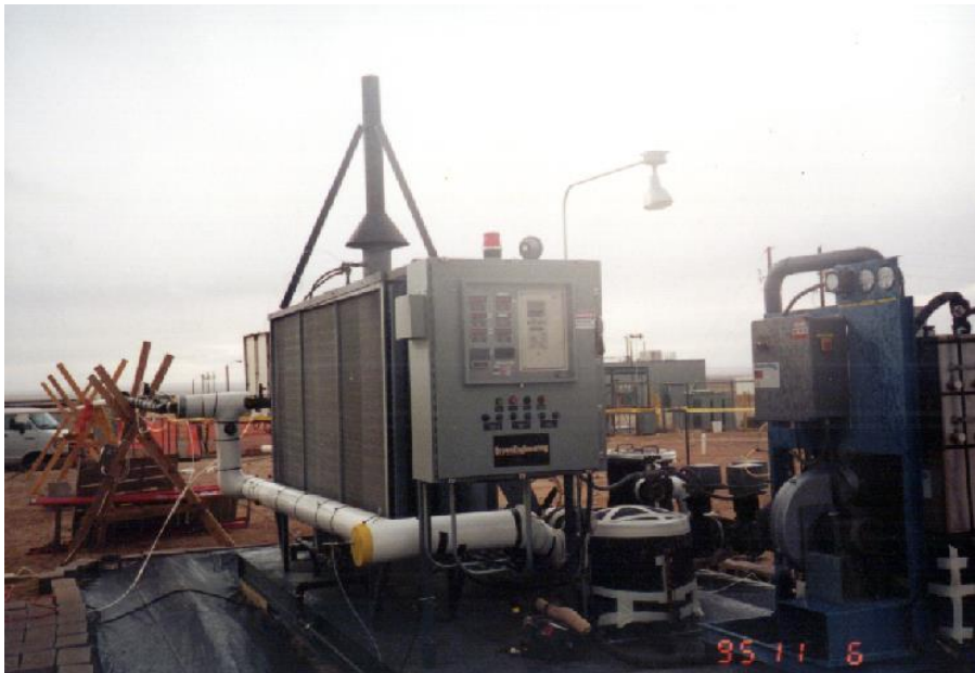
Vapor Extraction System
