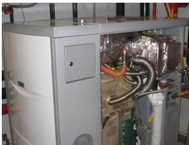
Figure 75: Peak Heater Module in Integrated Test Rig
