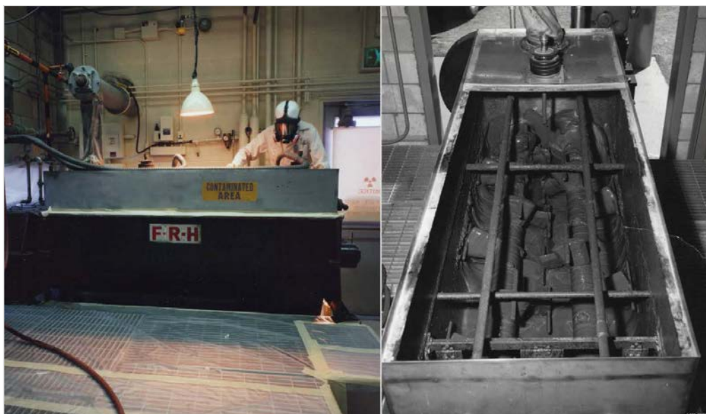
Figure 4. Pug Mill for Cementing Wastes at Building 21-257
