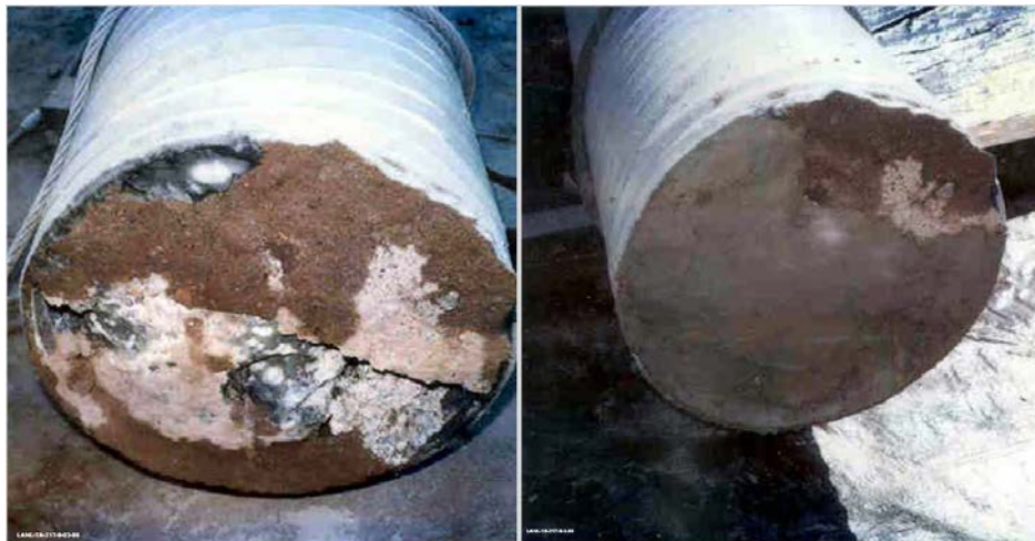
Figure 13. Damaged End of CMP Before and After Repair
