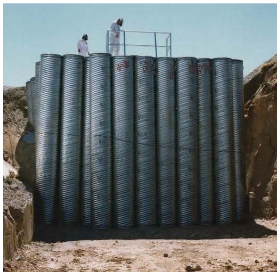
Figure 7. CMPs In Retrievable Waste Storage Area at MDA T
