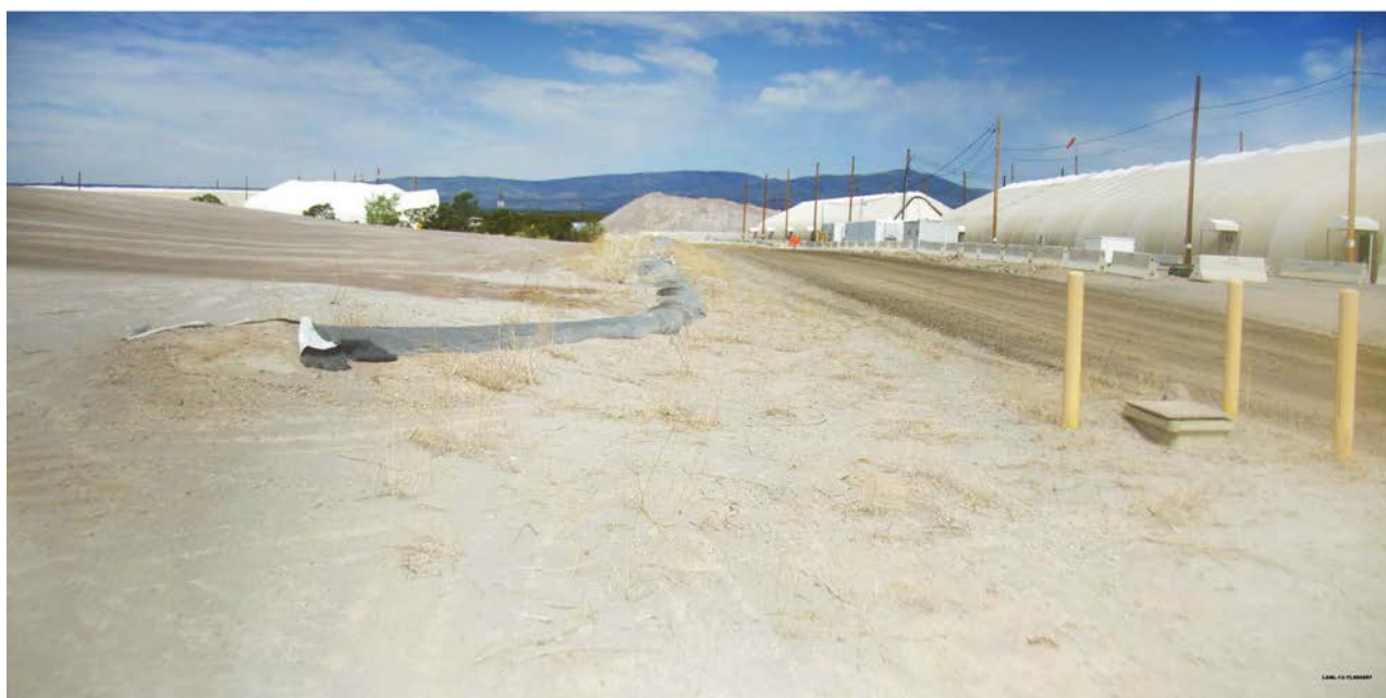
Figure 17. Photo of Ground Surface above CMPs in July 2013
