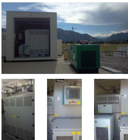
Figure 19. System Installation at NREL Facilities
