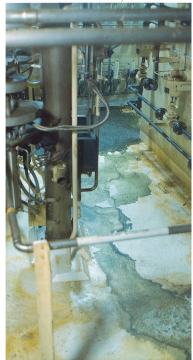
Spill at Processing Facility
