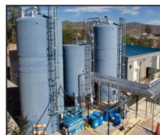
Sanitary Effluent Reclamation Facility
