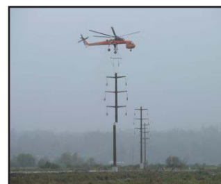
Additional 115kV Transmission Line
