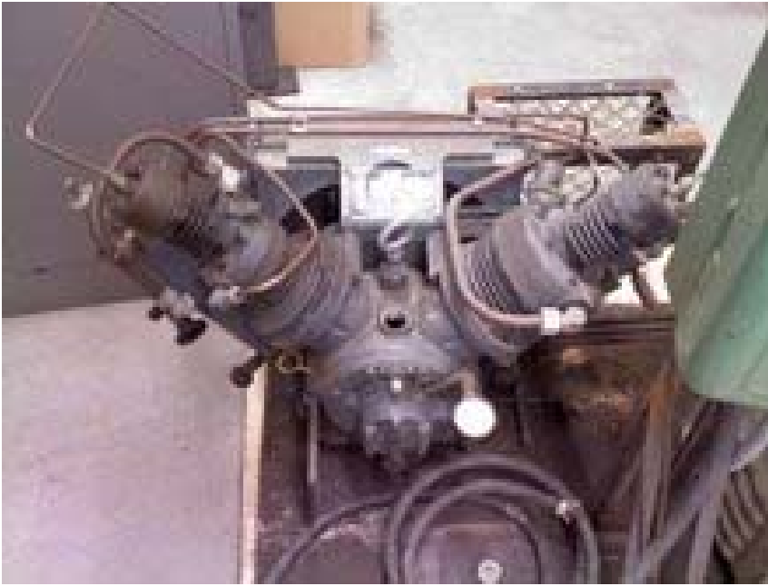
Figure 179 Four stage piston-type Joy compressor with the bottom two stages 1 and 2 not used in this experiment
