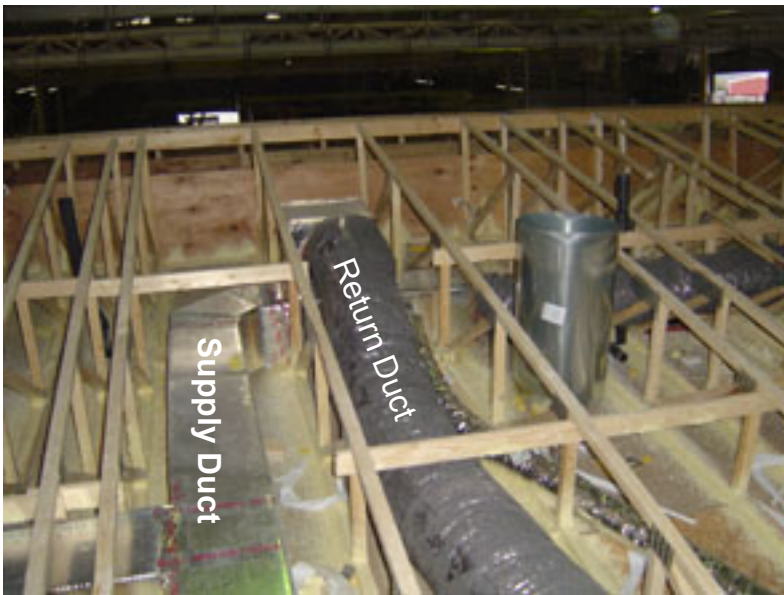
Exhibit 3.15: Supply and Return Ducts in Attic
