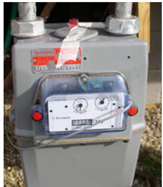
Exhibit 3.28: Gas Flow Meter
