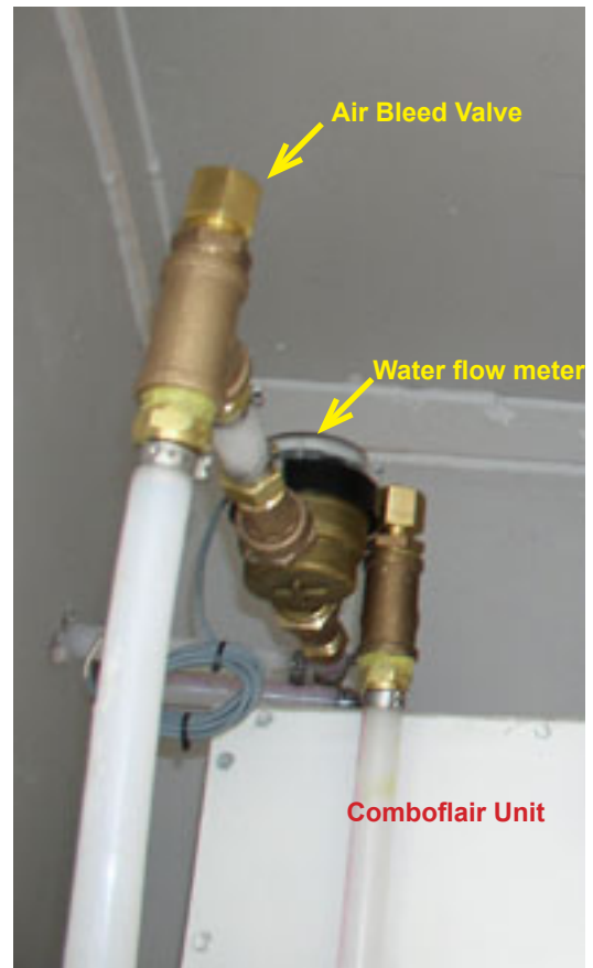
Exhibit 3.27: Water Flow Meter
