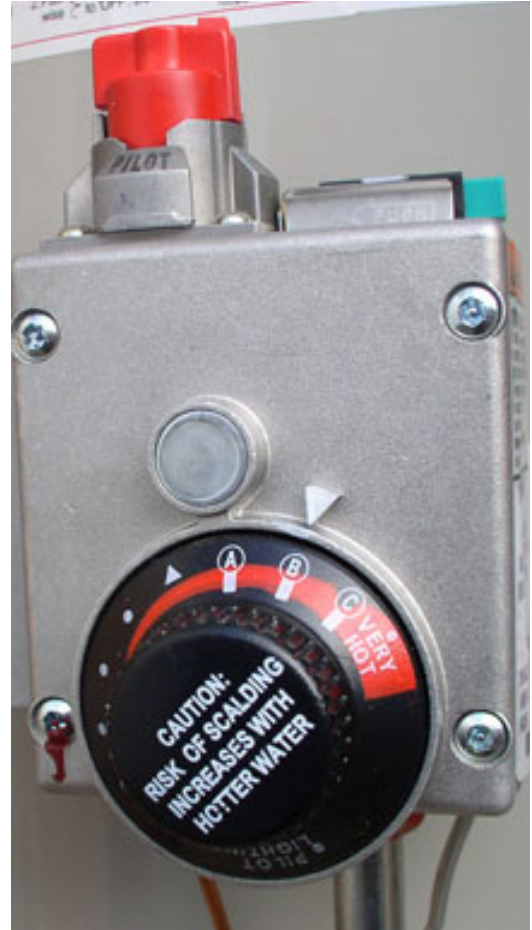
Exhibit 5.1: Typical thermostat for water heaters does not have temperature markings.
