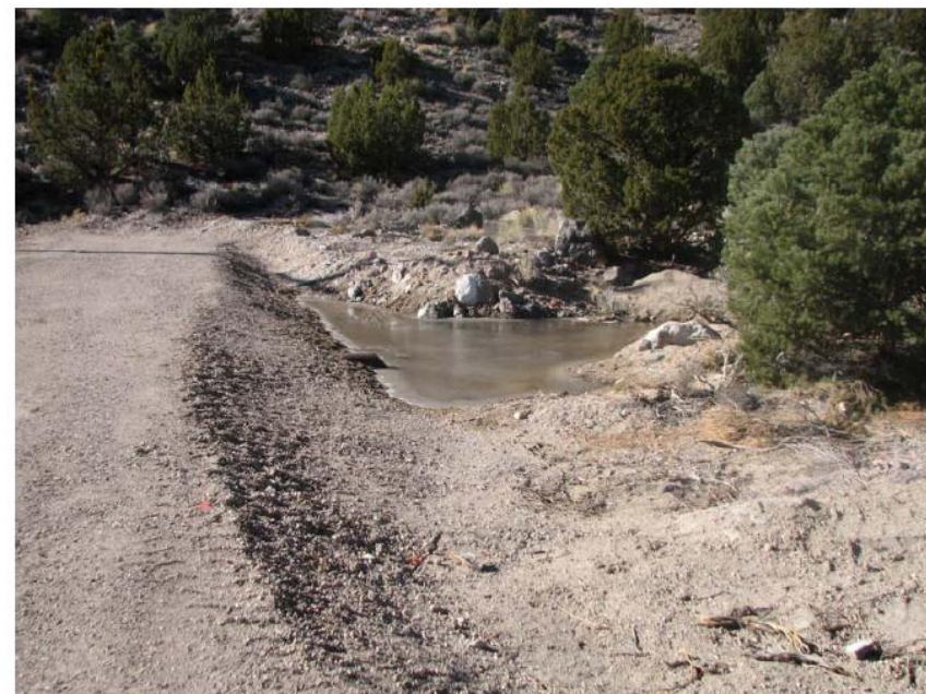
Photograph 4. Ponding behind Upper Berm (12/11/2008)
