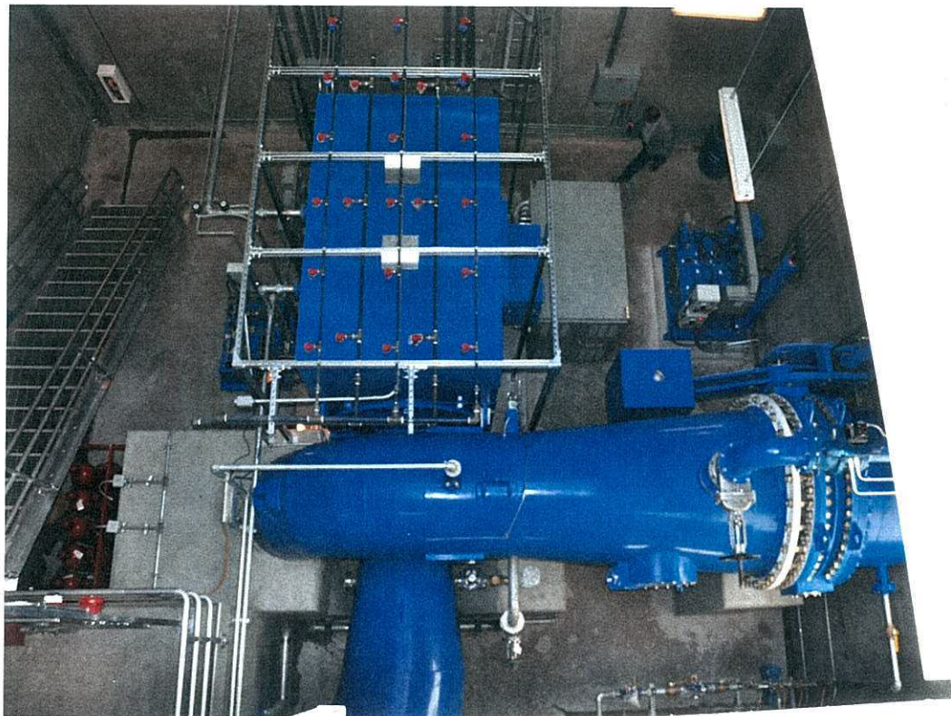
Abiquiu plant interior of new power house and low flow turbine-generator equipment - 21 April 2011.
