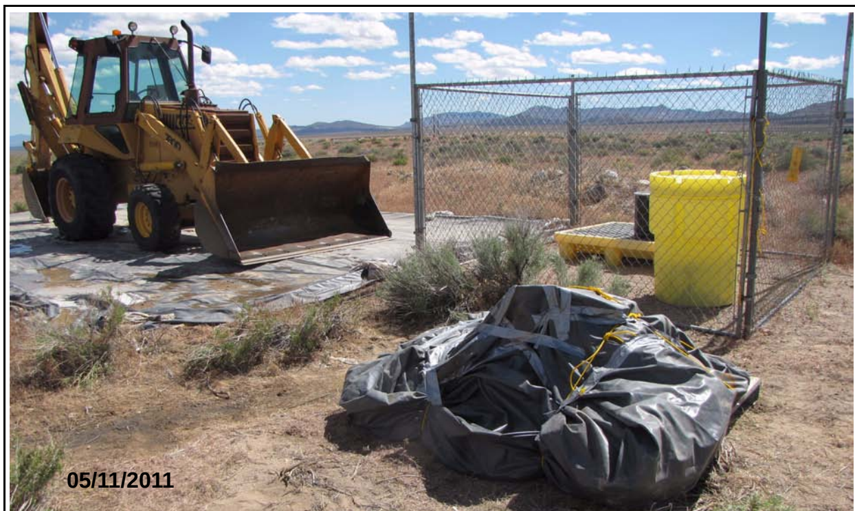
Figure D.1-3 CAS 02-08-02, Waste Dump and Burn Area, Melted Lead Staged and Wrapped on Metal Pallet
