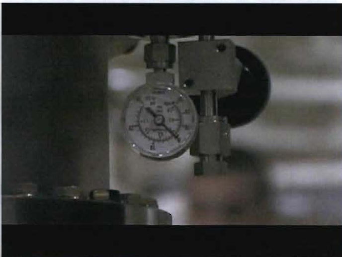
FIG. 6: VACUUM/PRESSURE GAGE AT ZERO DOCUMENTING OPEN VALVE.
