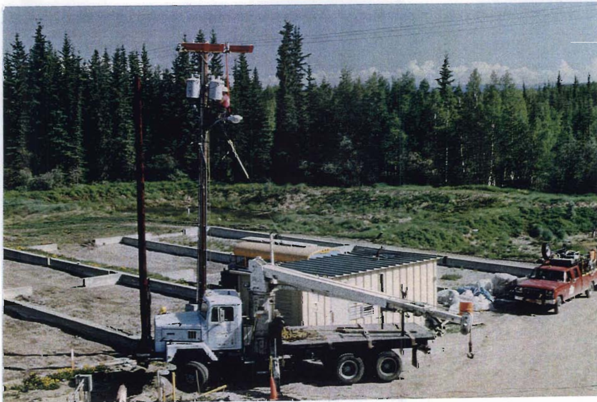
FIGURE B.4. Wastewater Treatment Plant. Rectangular concrete-lined containers are the sludge drying beds. The spill ponds, WP32, are located beyond. Note that the ponds are separated by a berm and culvert seen above and left of the red truck.
