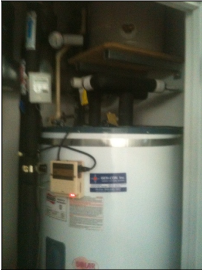
Figure 67. Drain-back and solar tanks
