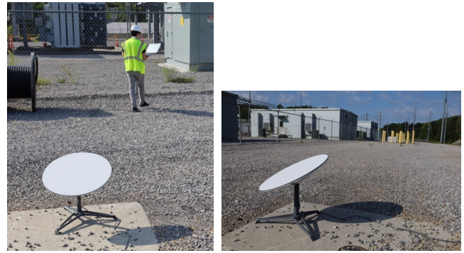
Fig. 8: Starlink transceiver deployed at utility substation.
