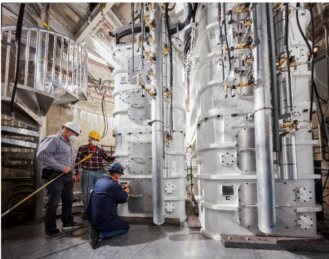
Figure 2: Two of MJOLNIR's six pulsed power pressurized towers.
