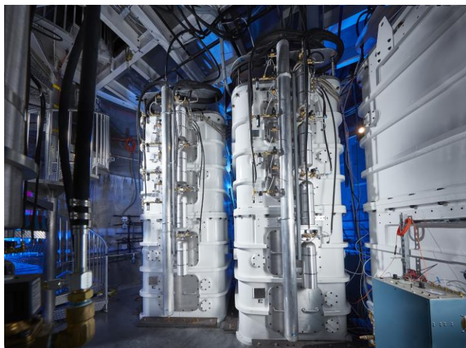
Fig. 2. Three of MJOLNIR's Marx bank "towers," containing 1 MJ stored energy at maximum voltage (100 kV).
