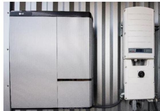
Figure 4. Residential battery and inverter.
