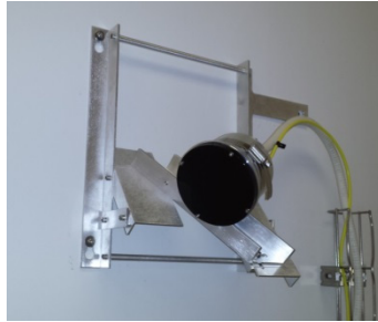
FIG 5. The installed 15.9m PMT nTOF detector with black lead shielding.
