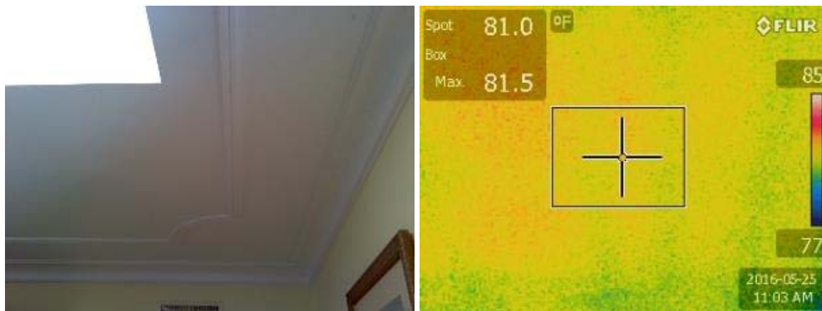
Figure 4: Digital and Infrared Picture of West-facing Ceiling and Wall
