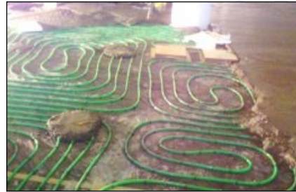
Figure 4: Radiant floor cooling system
