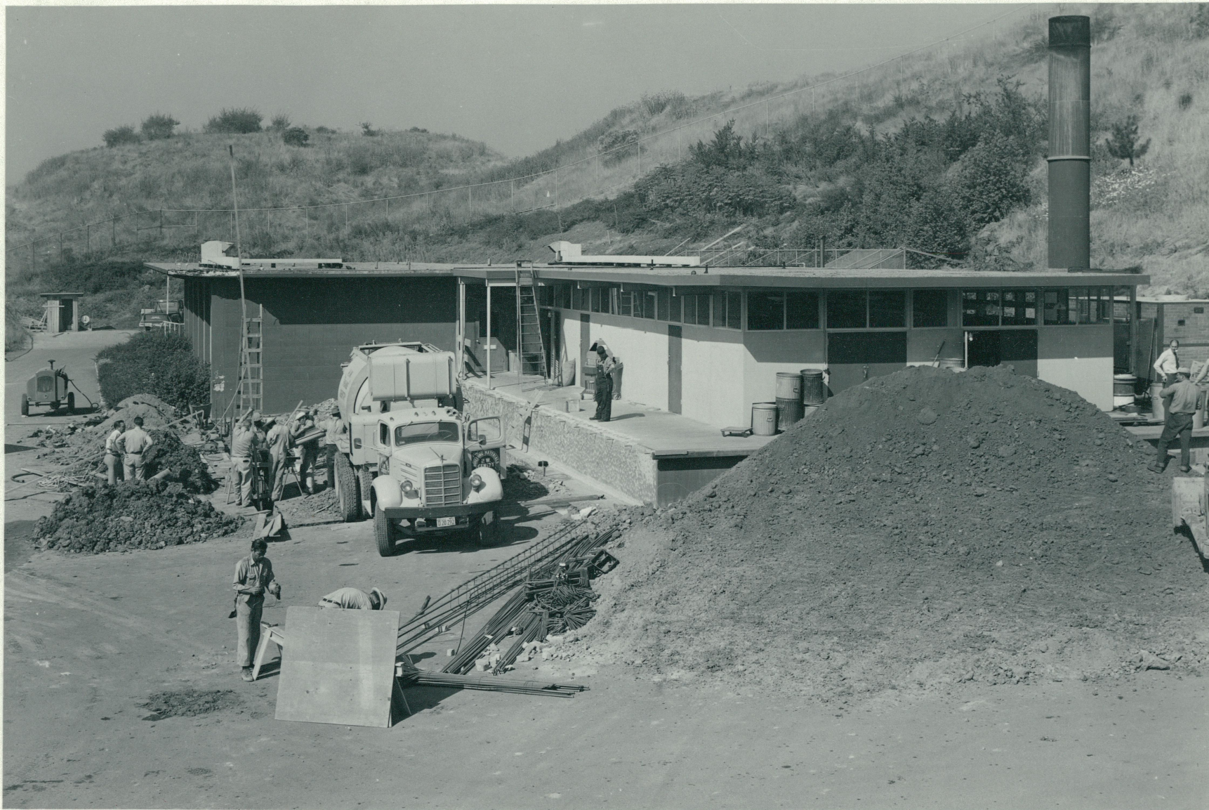
University of California Radiation Laboratory Animal House Addition Bldg. 55 Date: September 28, 1956 7 % Complete Leo S. Holm Subcontract No. 103
