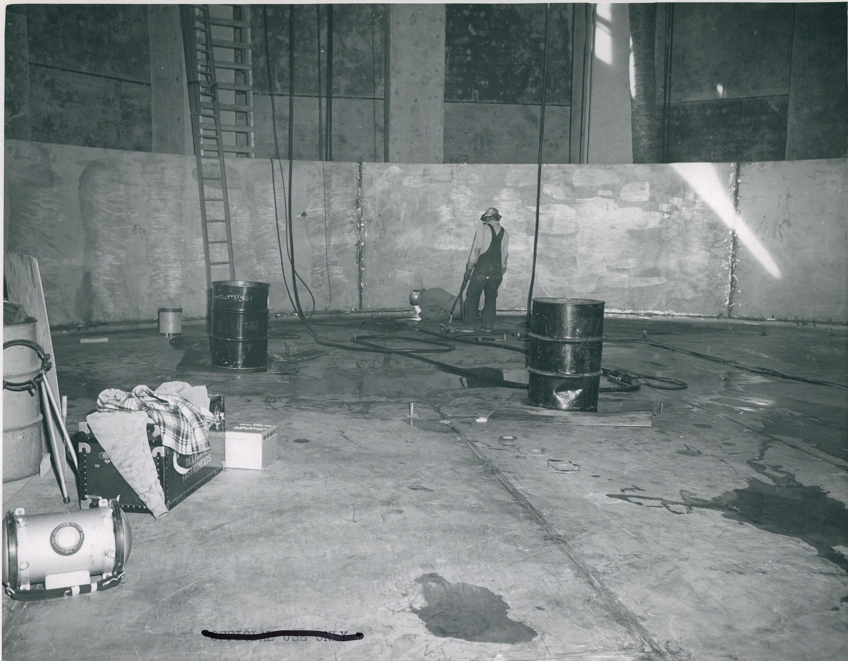
CONFIDENTIAL USE ONLY CPP - Welding on Tank WM-183 inside tank enclosure. Tank WM-183, 54.2% complete. J. F. Pritchard and Company, Contract AT(10-1)-744 Idaho Operations Office, March 21, 1955
