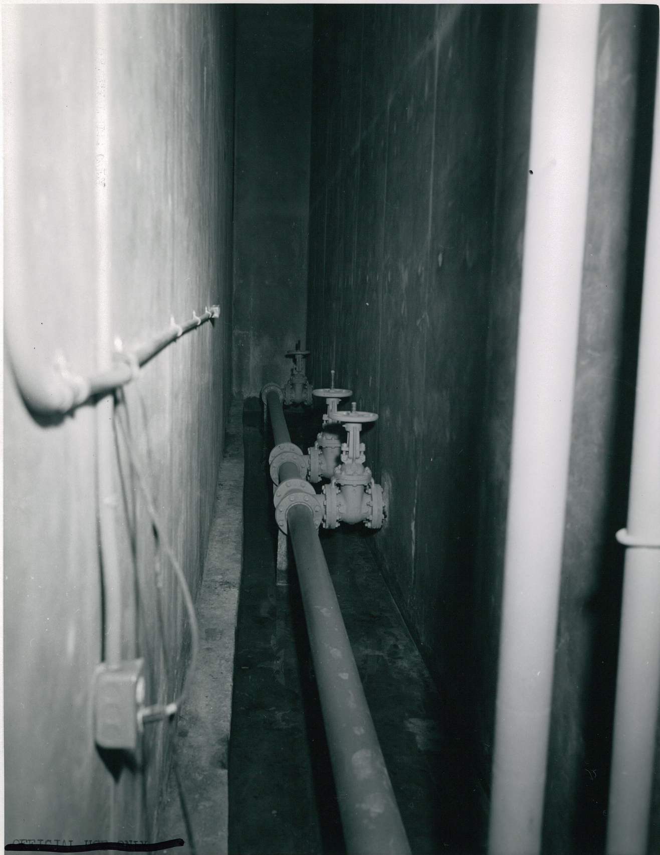
CONFIDENTIAL MTR - Piping and valves in pipe pit of Gamma Irradiation Facility Building Gamma Irradiation Facility Building 100% complete Arrington Construction Company - Contract AT(10-1)-758 Idaho Operations Office - March 21, 1955
