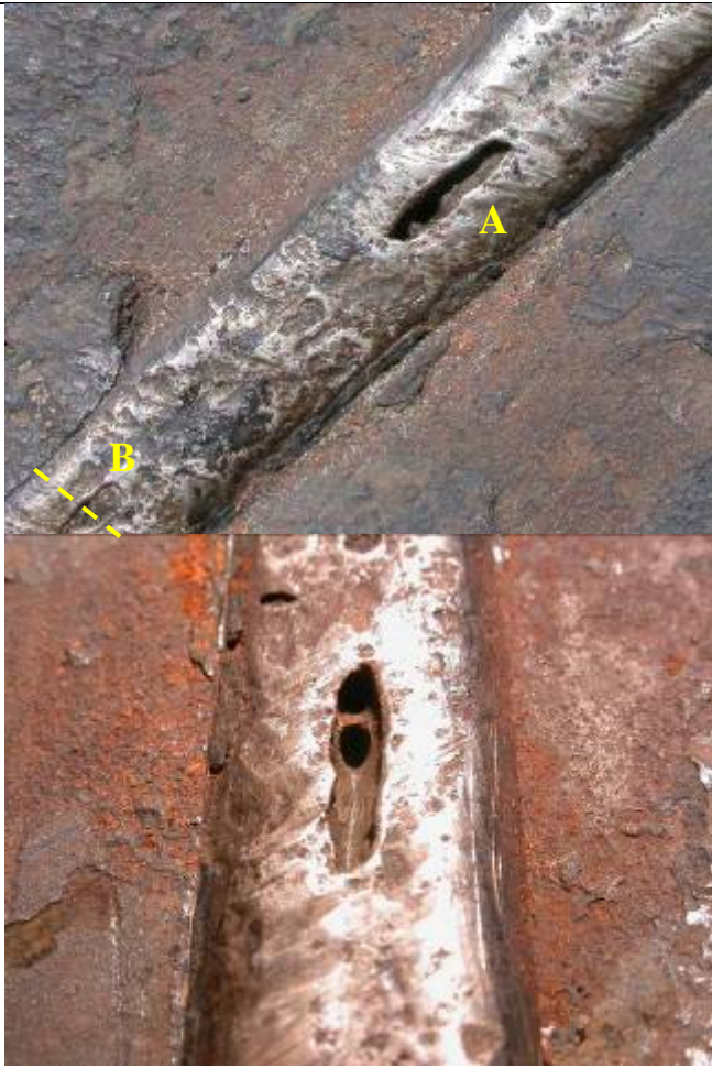
Figure 3: Other defects along the weld
